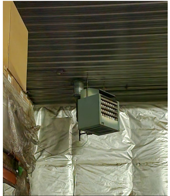
South Unit Heater Parking Barn
